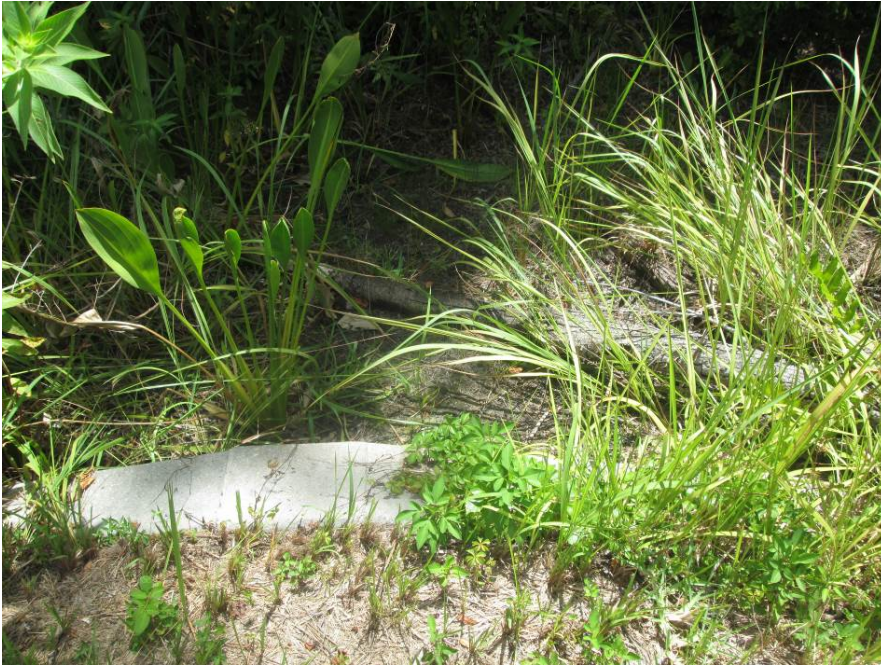
Item 1 - Pond 49 - Remove dead tree laying across outfall at headwall
