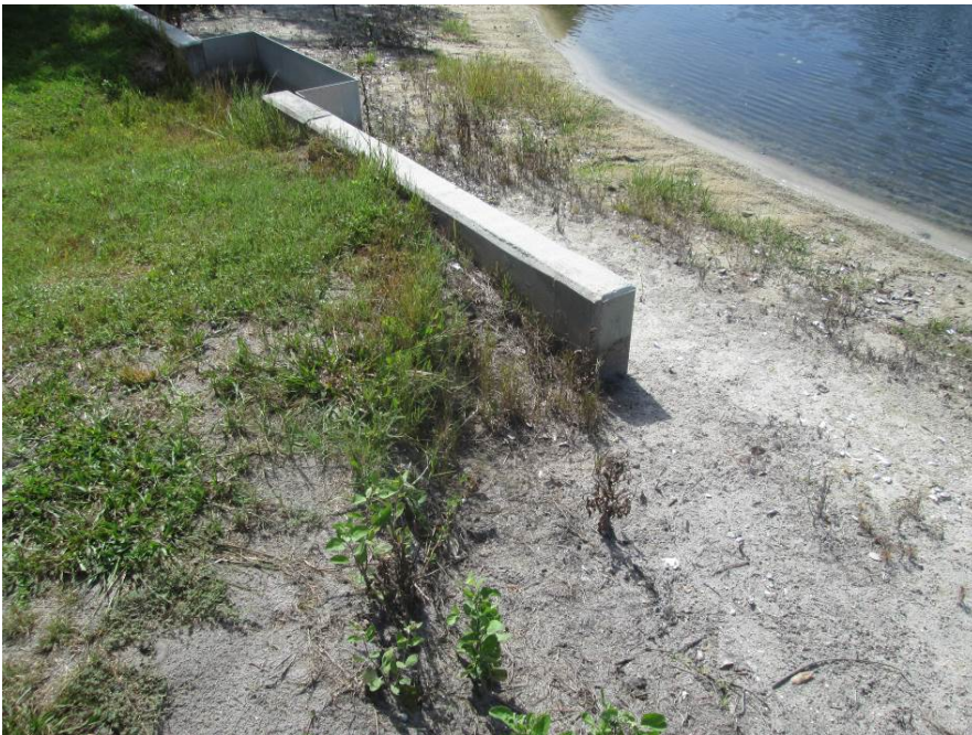
Item 6 - Pond 40 - Minor erosion on east side of weir - monitor
