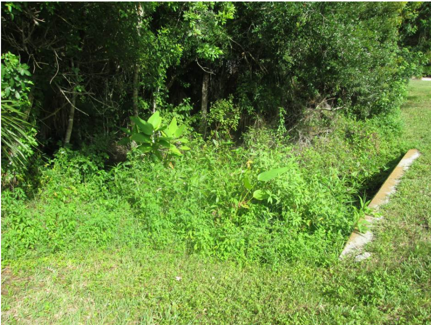
Item 11 - Wingspan, s/o of Tara Preserve – Remove 15' veg. at east headwall
