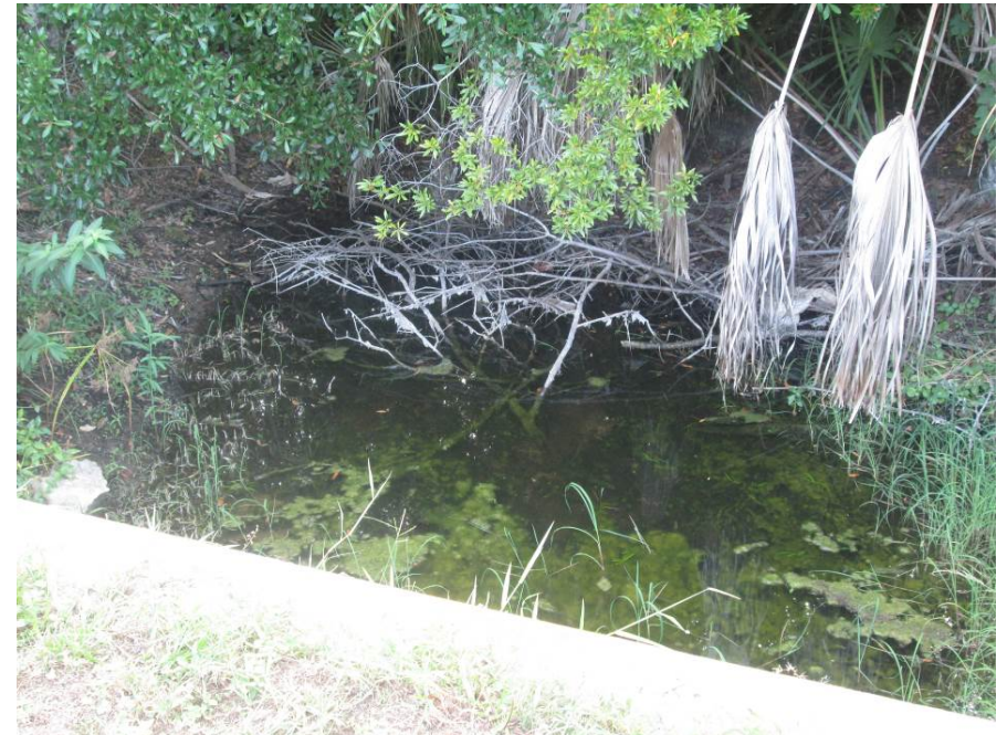
Item 10 - Southern Wingspan Way – Remove dead debris at west headwall
