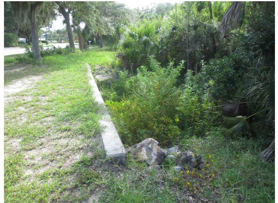
Item 13 - East Tara Preserve Ln – Cut back 15' veg on north side of headwall
