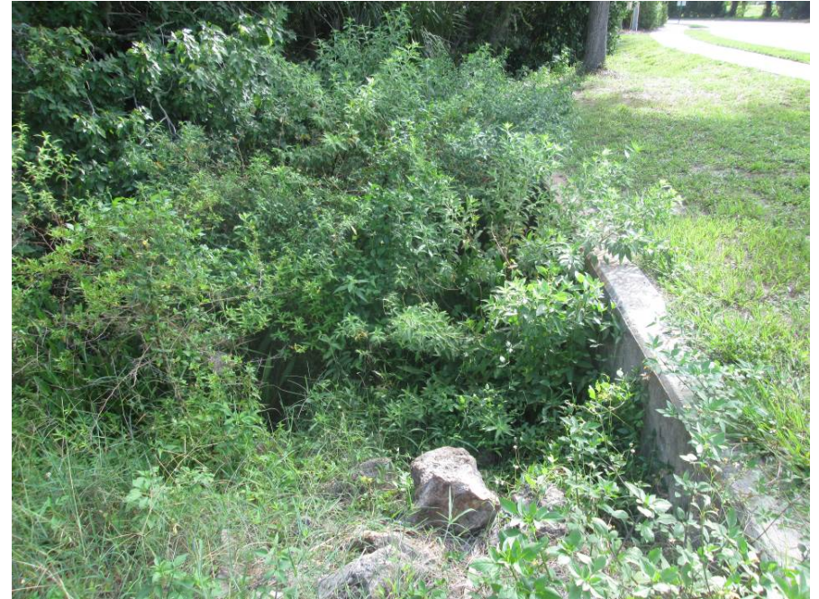
Item 13 - East Tara Preserve Ln– Cut back 15' veg on south side of headwall
