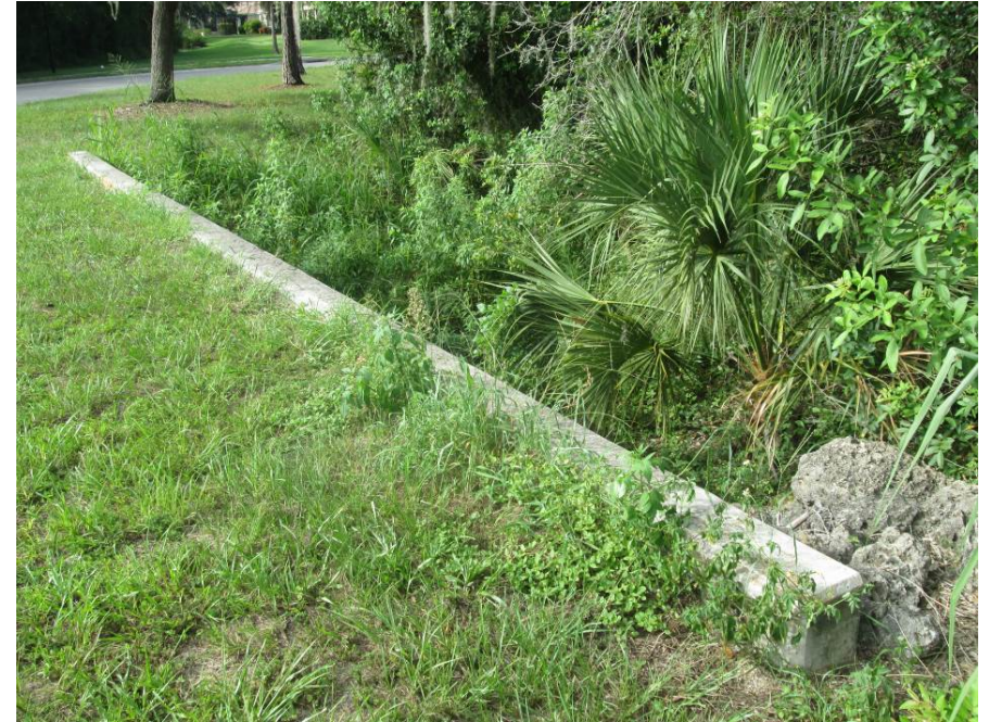
Item 18 - Wingspan near Pond 9 – Remove 15' vegetation at east headwall
