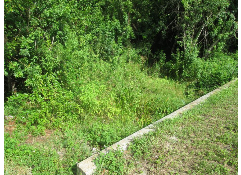
Item 10 - Southern Wingspan Way – Remove debris 10' from east headwall
